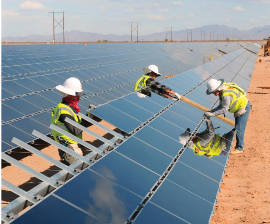
First Solar employees work on the solar power station in Blythe, Calif. (Credit: First Solar)
